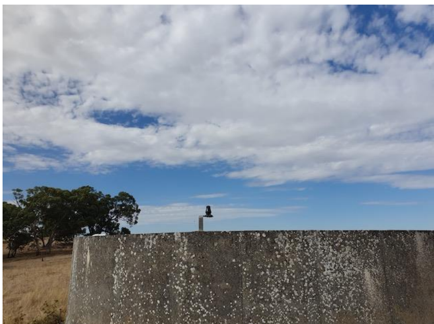
Figure 2: T35 Tank Level Sensor
