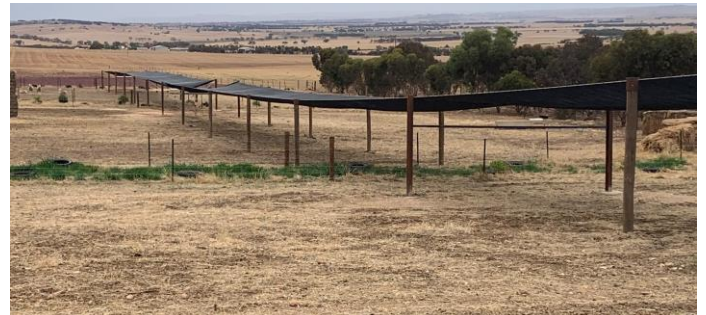
Schutz's heavy-duty shade across the containment pens – materials purchased and installed themselves.
