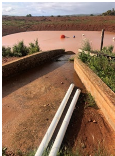
Storm water pipes carry runoff from liner to concrete inlet of dam.
