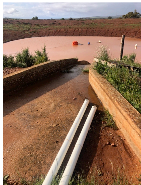
Storm water pipe enabling water flow into the dam causeway from the lined catchment
